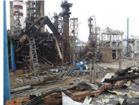
Undetected corrosion – hydrocarbon release
